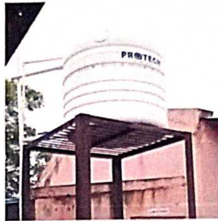
Fig No.2 Water storage
